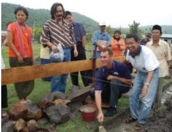
Chris Dickson (center), a JIS teacher, lends a ceremonial hand to the laying of the foundation for the library with Arian Ardie ('79, in batik).
